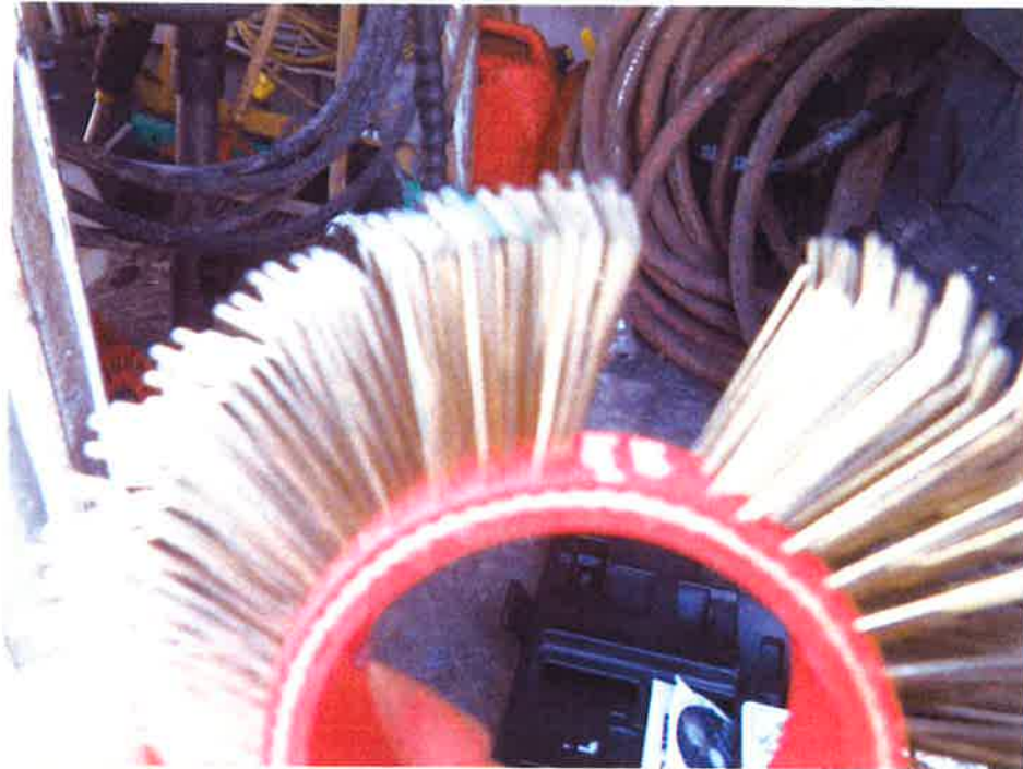
Image #9. May 4th. This unit removes failed paint and rust while imparting a profile to the surface.
