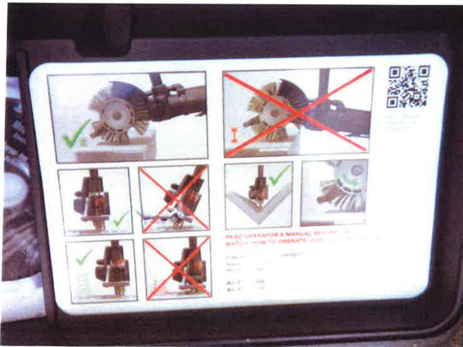
Image #8. May 4th. Surface preparation is being addressed using a 'bristle blaster'.
