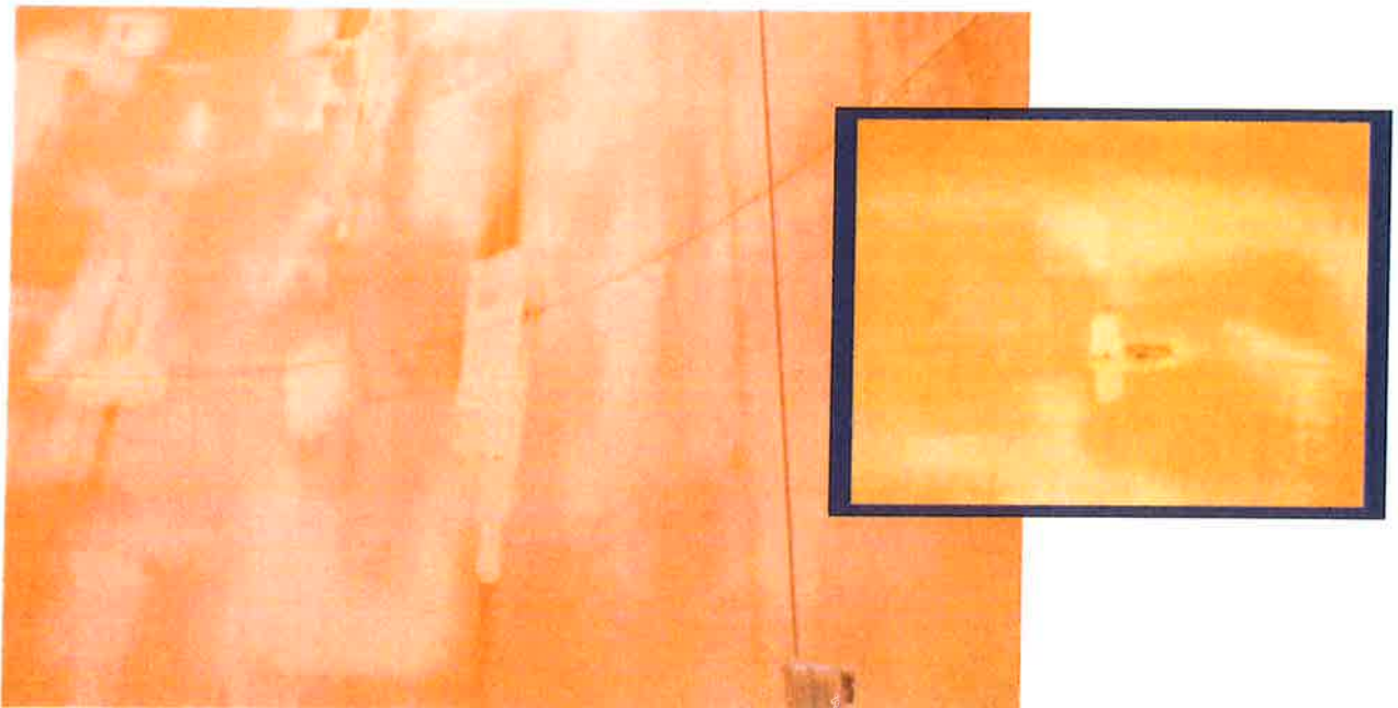
Image #4. May 3. There are a number of sites that have been previously repaired. Most of these are intact, while some have corrosion staining visible within them.
