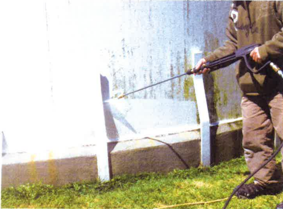
Image #18. May 6th. Contractor using high pressure water washer to remove mildew.
