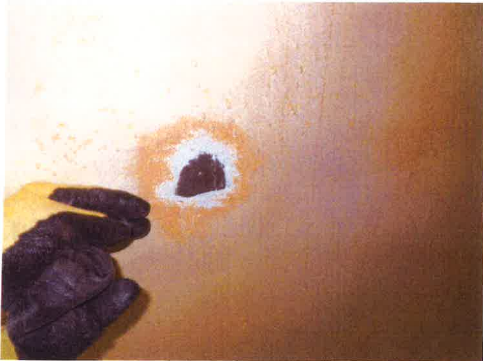
Image #13. May 4th. Small repair sites are hand abraded to feather-edge before bristle blasted to give profile to the surface.
