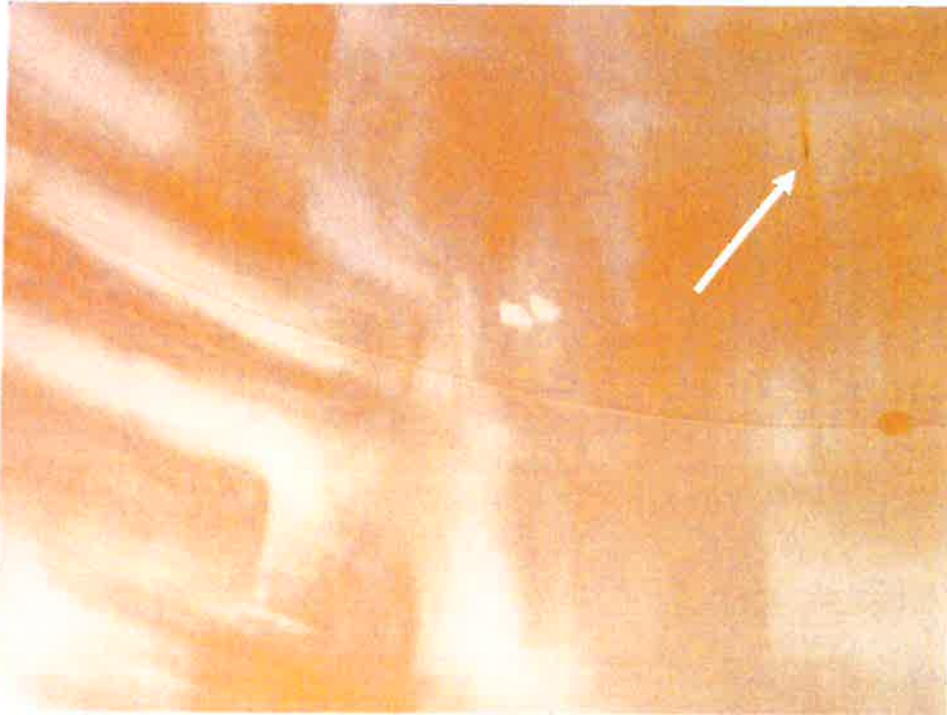
Image #7. May 3. There are a number of small corrosion sites visible.
