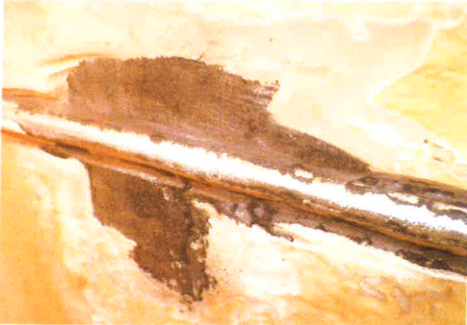
Image #11. May 4th. Note surface profile visible in the bare steel, which is ideal for the requirements of the coating at application.
